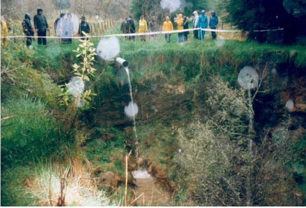
Gully erosion protection works pipe with a piddle (and yes those are spots of rain on the lens)
