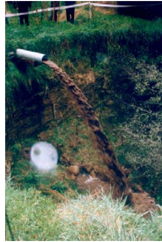
Gully protection works pipe with a good gush only minutes after the pic on left.
